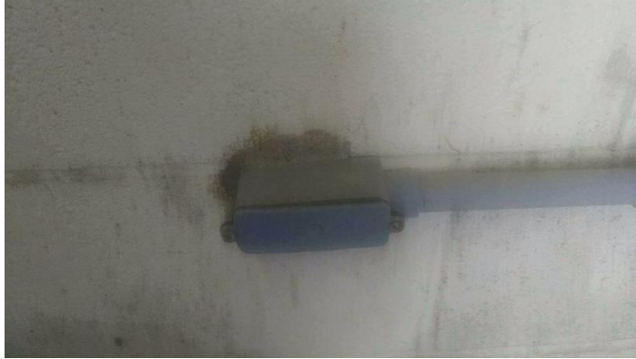
Chlorine room wall patch #1
