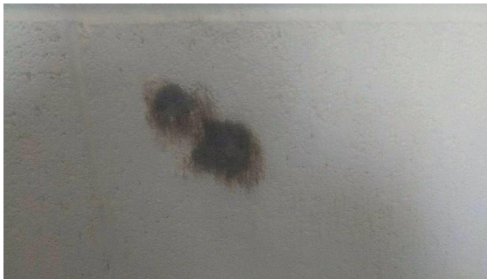
Chlorine room wall patch #3
