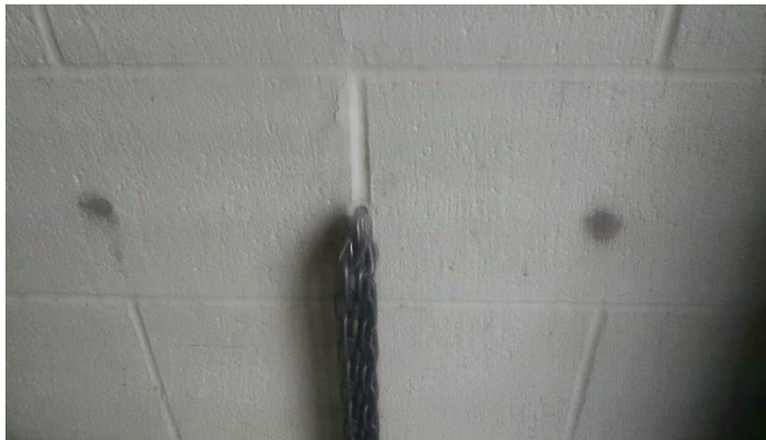
Chlorine room wall patch #2
